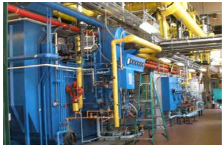
Farmingdale College - Central Utility Plant
