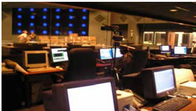
Command and Control Facilities
